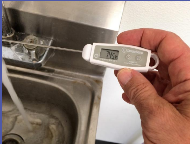
Hot water < 100°F
